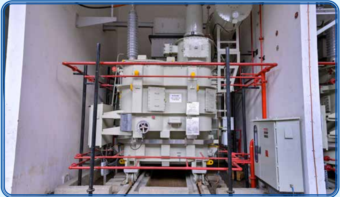
Transformer in Transformer Hall
