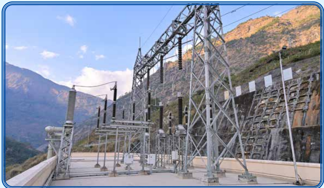
220kV Outgoing Switchyard
