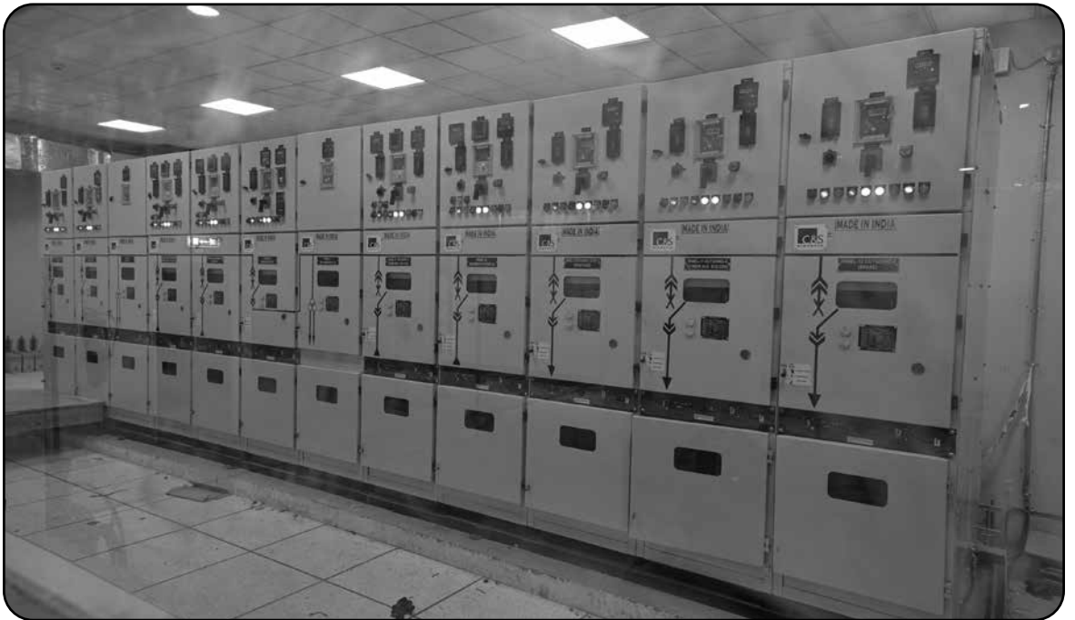
11kV Control Panel
