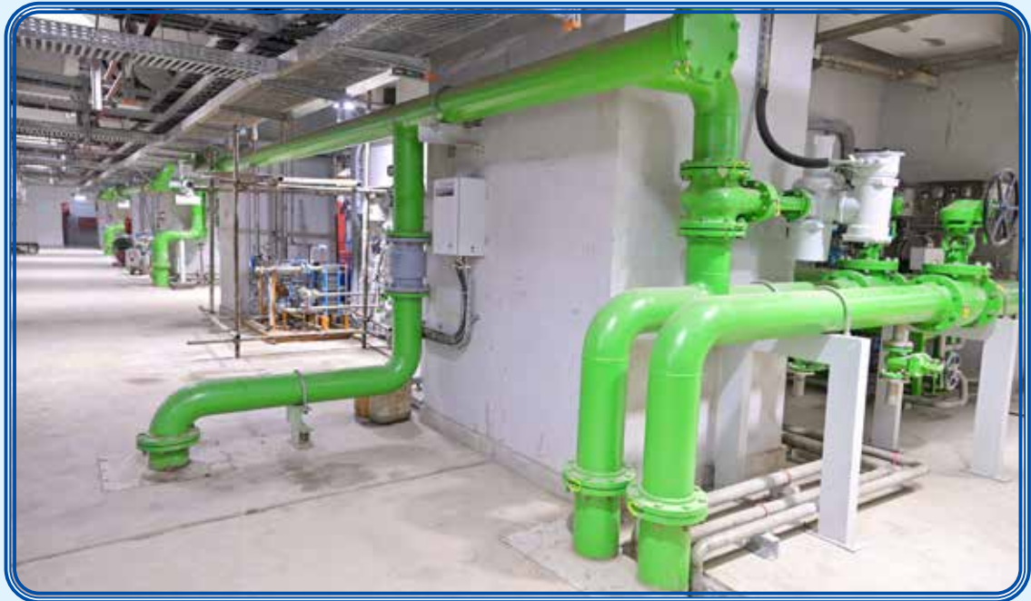
Cooling Water System
