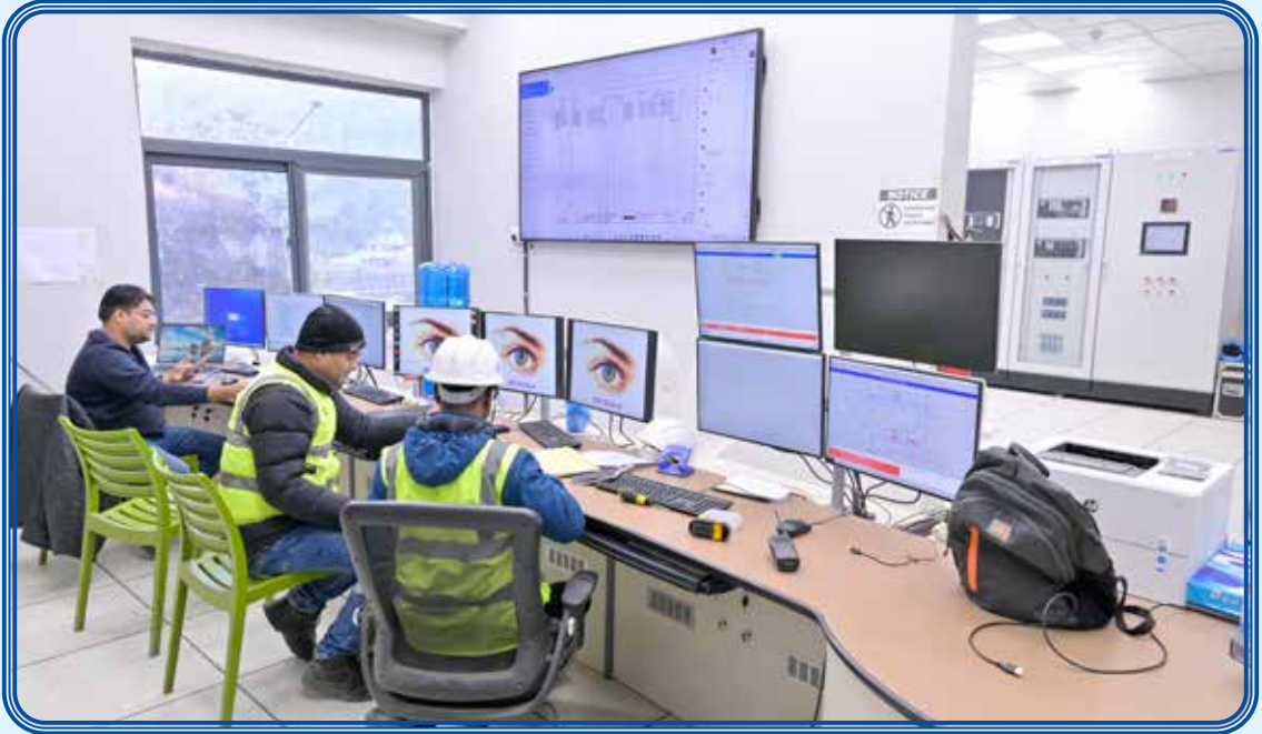
Computerized Control System
