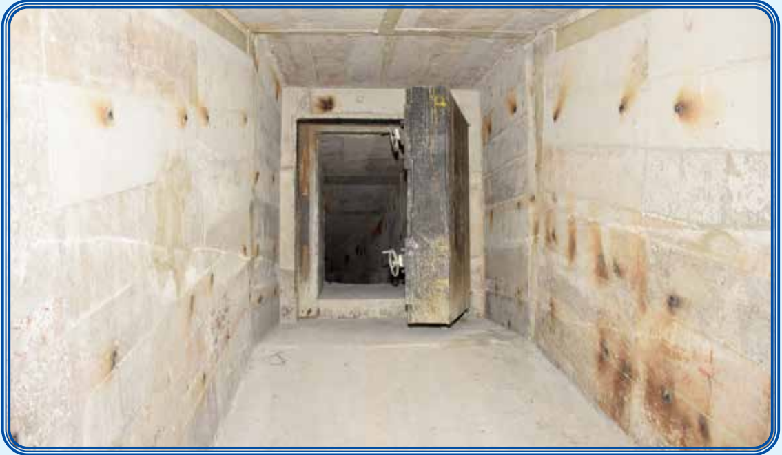
Adit-2 Bulk Head Gate
