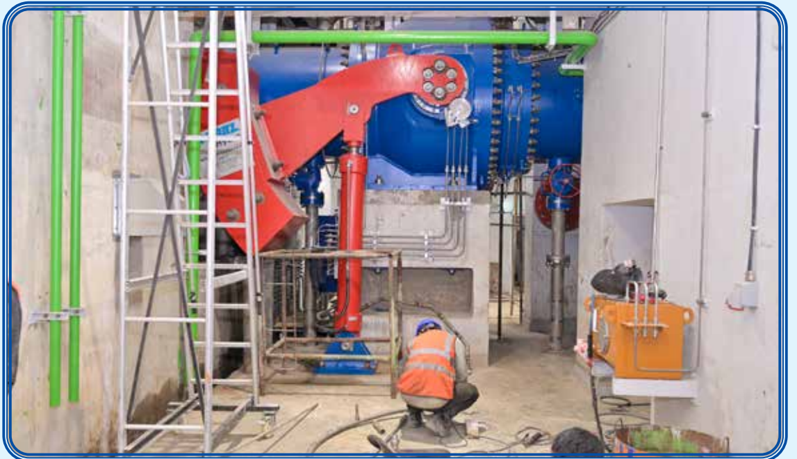
Main Inlet Valve
